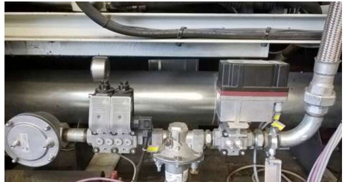
CHP for generating electricity and heat
